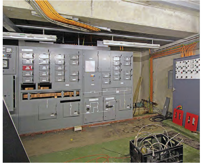
The generator control panels and the main electrical switchboard
